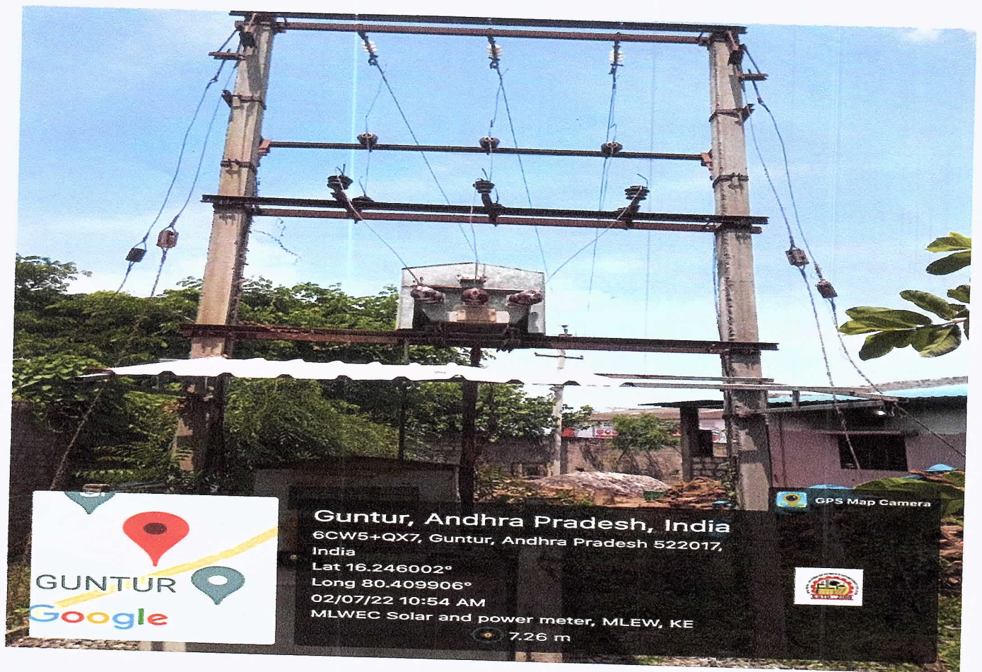
Solar and Power meter at college campus
