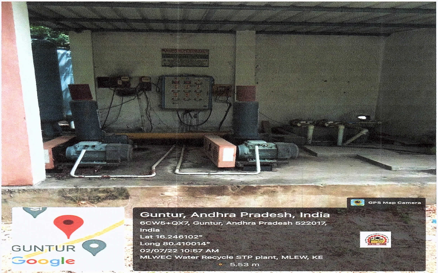
Waste Water Recycling STP
