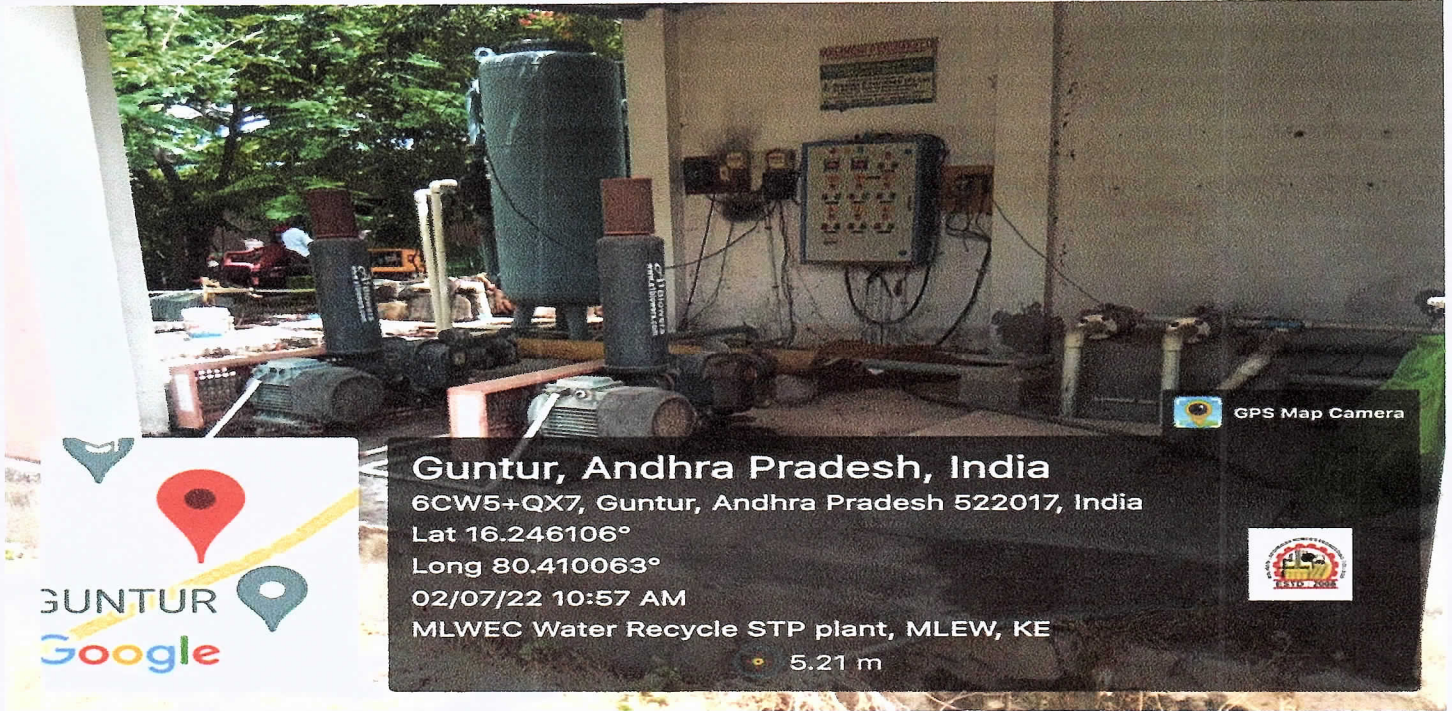
Waste Water Recycling STP
